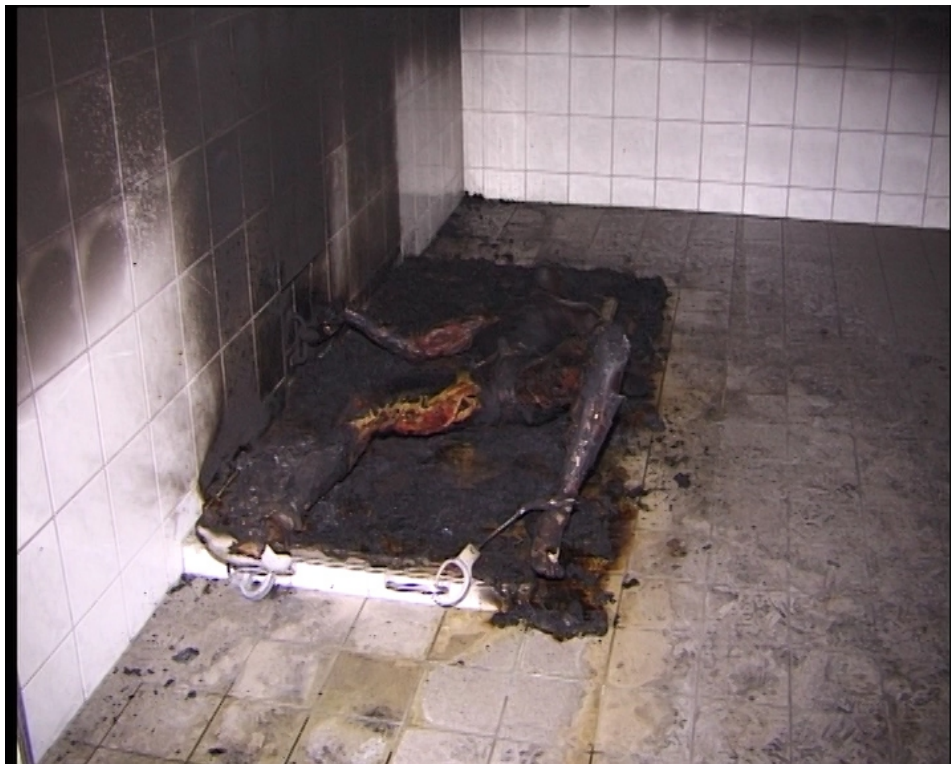
Image showing fire damage from Detention cell 5, Dessau Police Station
